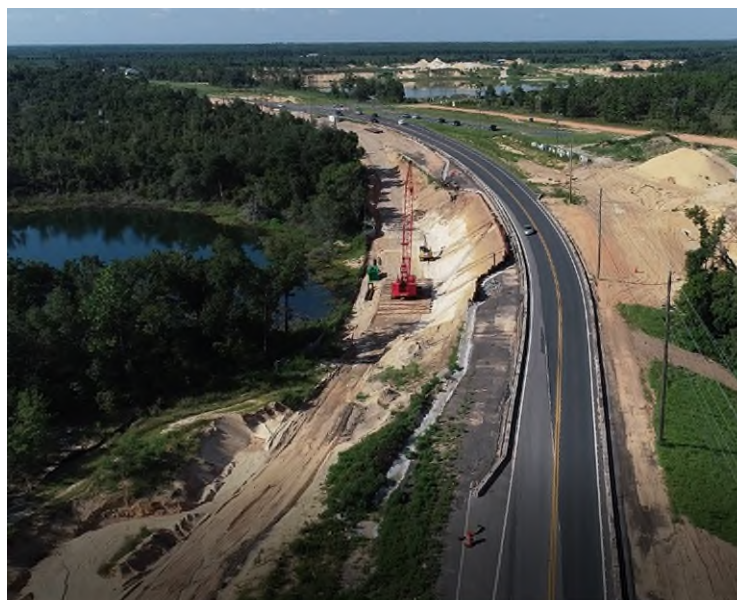
S.R. 77 Widening from the Bay County line to north of County Road (C.R.) 279 (Moss Hill Road) (District 3)
