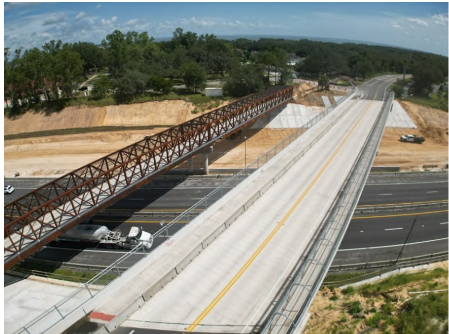
Mainline Widening from Clermont/State Road 50 to Minneola/Hancock Road (Both) (Florida's Turnpike Enterprise)
